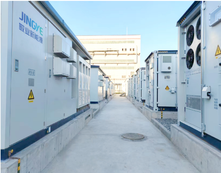
华西特钢 15MW/30MWh 储能电站实景图 Huaxi Special Steel 15MW/30MWh Energy Storage Power Station RealScene
