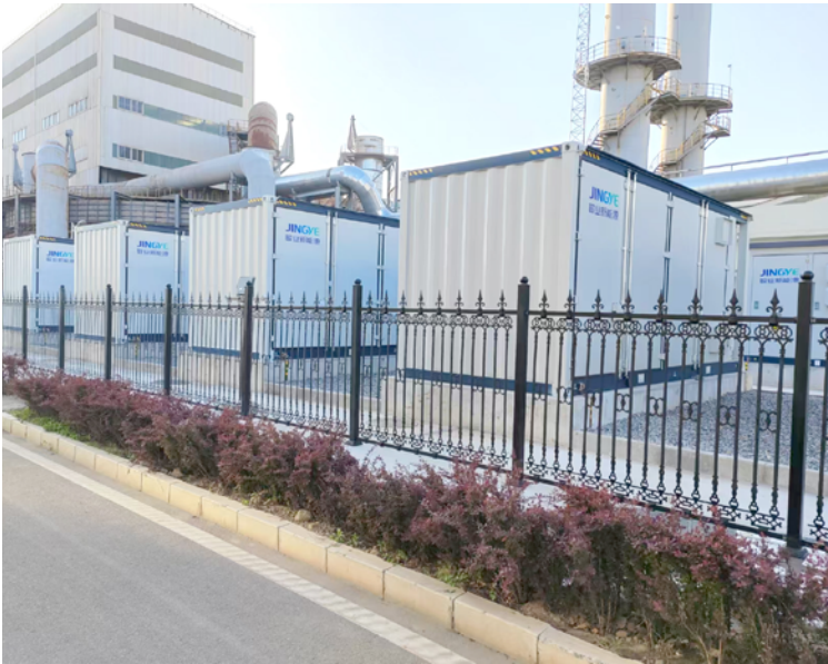
江苏敬业 50MW/100MWh 储能电站实景图 Jiangsu Jingye 50MW/100MWh Energy Storage Power Station Real Scene
